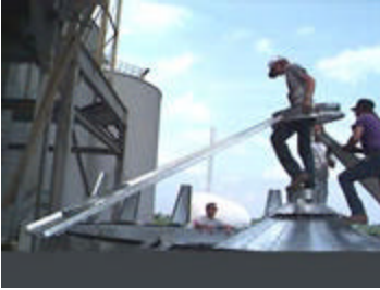
Photo 4. Bring two opposing tower roof sheets to the tower roof center collar.
